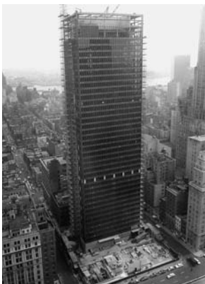
IMAGE SIXTEEN: Ludwig Mies van der Rohe. American, born Germany. 1886–1969. Seagram Building, New York. 1954–58. Construction photograph showing steel frame. Photo: House of Patria. The Mies van der Rohe Archive. Gift of the architect
